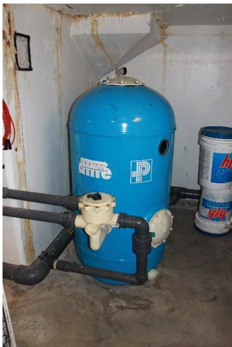
Bilde 37 Kullfilter, modent for utskifting.
