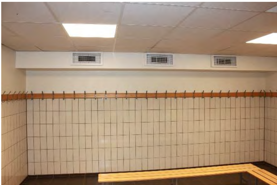
Bilde 22 Garderobene trenger full rehabilitering
